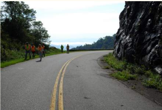
The pavement has been damaged by fallen rock and the roadway width is impacted by the encroachment of vegetation. (Credit: Dan Nabors)
